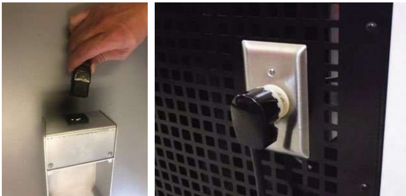
Figure 5: Electrical cable and cabinet power receptacle
